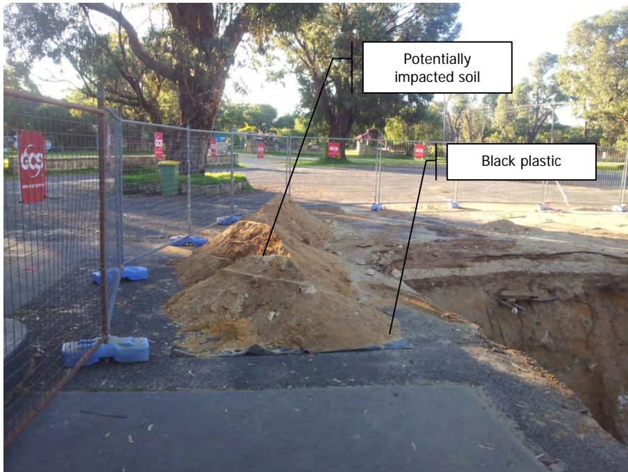
Minor quantity of temporarily stockpiled potentially impacted soil – view to the north
