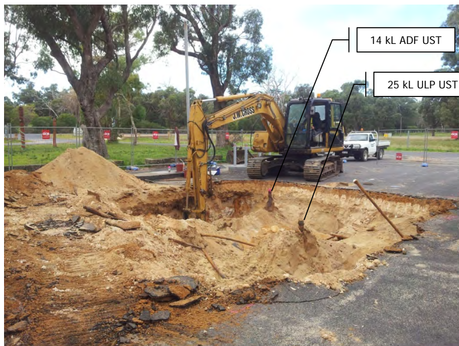
Exposing the 14 kL ADF and 25 kL LRP USTs – view to the south-east
