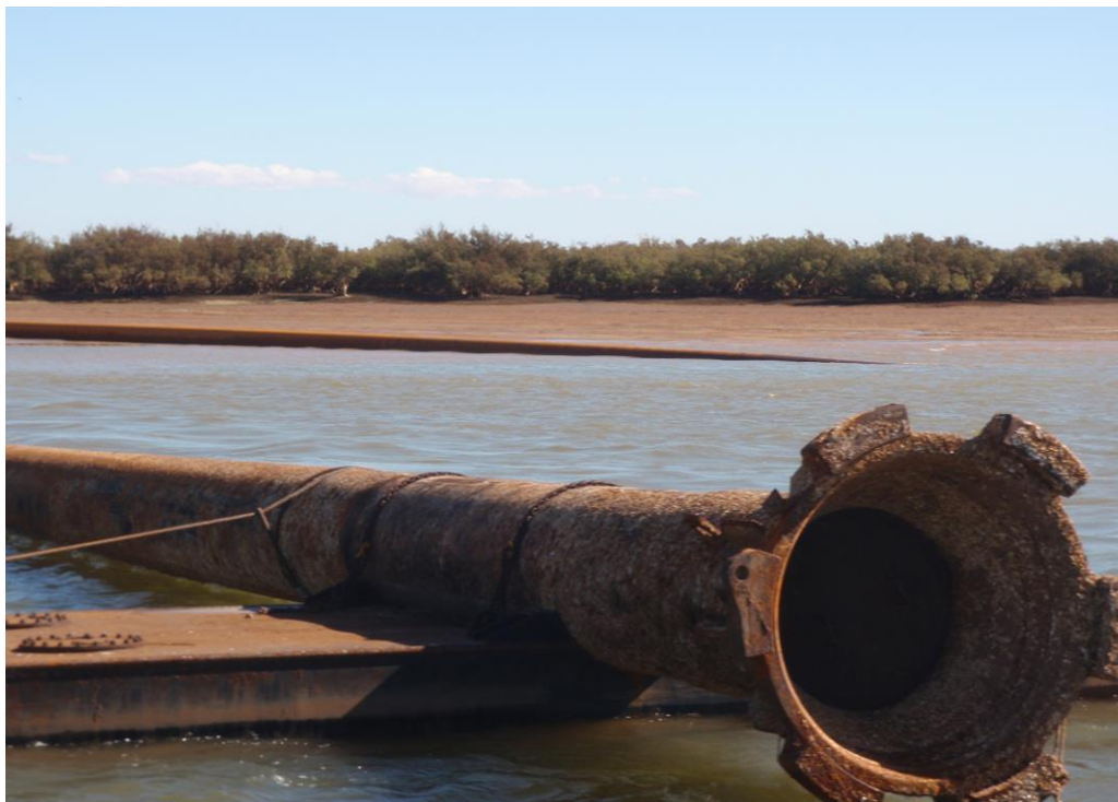
Figure 3: Cutter suction pipelines at DMMA H as part of BHPBIO's RGP6 expansion
