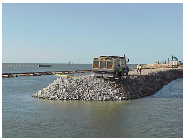
Figure 6: Aerial and ground-level views of a bund wall development similar to what is proposed for the Lumsden Point General Cargo Facility. Note that in these photographs, the core of the wall has been placed, with outer armour rock layers to be installed.
