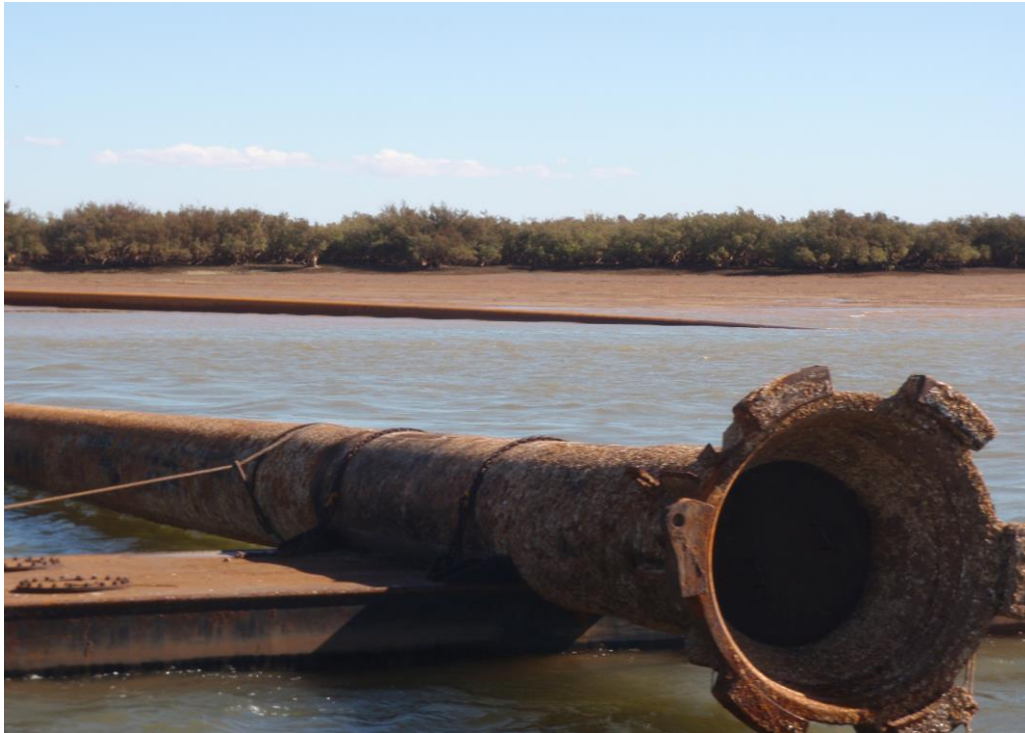
Figure 11: Cutter suction pipelines leading to DMMA C as part of BHPBIO's RGP6 expansion
