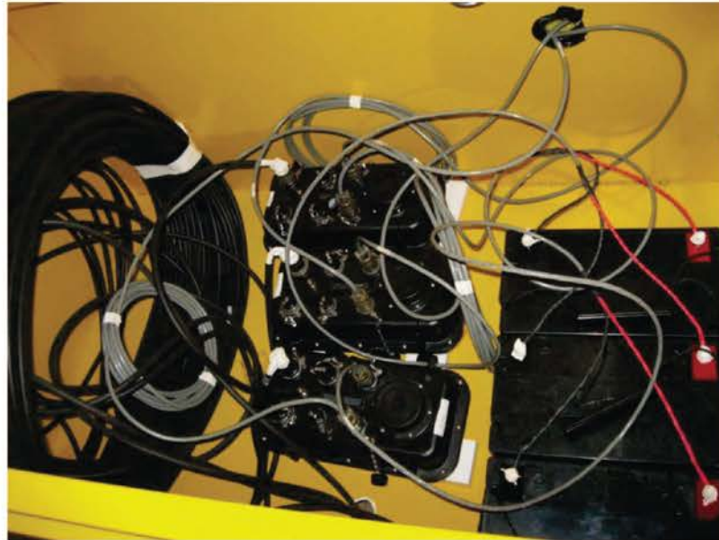
1.3 Inside the housing box showing electronics for data collection and power supply
