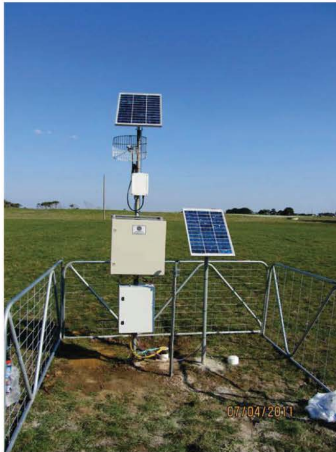
2.2 Example electronics housing with solar power and radio communication
